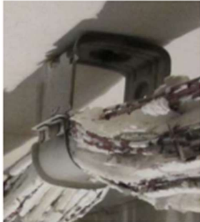
Fig. 5: Deformation during ceiling mounting
