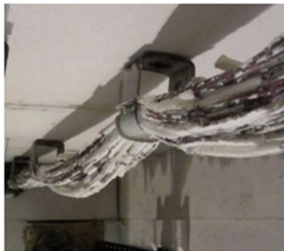
Fig. 7: Sagging cables after a fire load of 90 minutes
